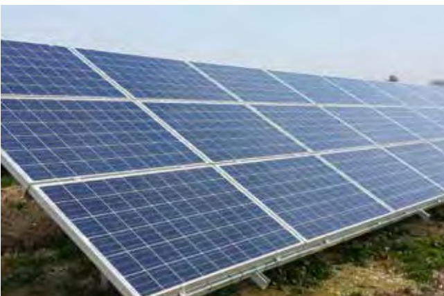
IRELAND Dale Farm, 4MW HEV 1500 + MV SKID
