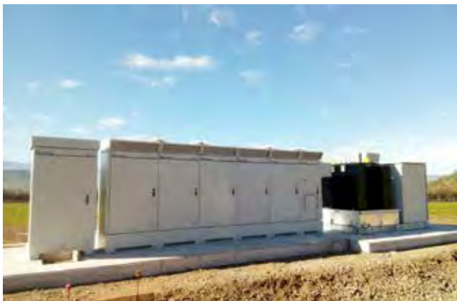
CHILE Santiago Solar, 115MW HEC PLUS + MV SKID
