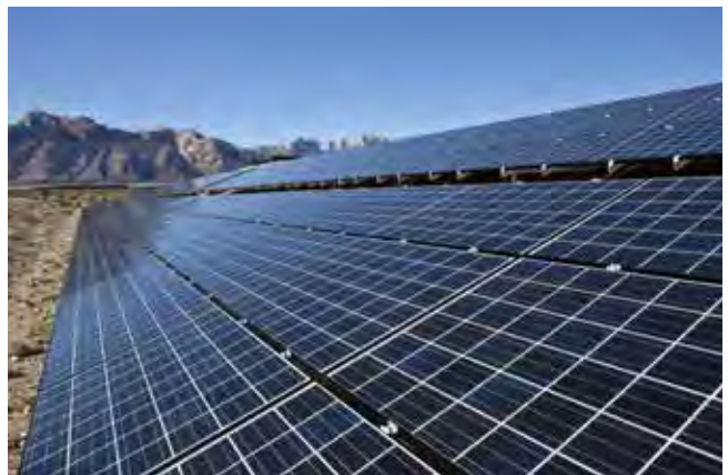
MEXICO Solem I & II, 175 + 165 MW HEC V1500 + MV SKID
