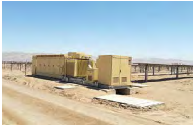
CHILE Uribe, 50MW HEC PLUS + MV SKID
