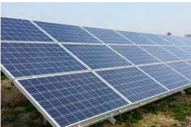
IRELAND Dale Farm, 4MW HEV 1500 + MV SKID
