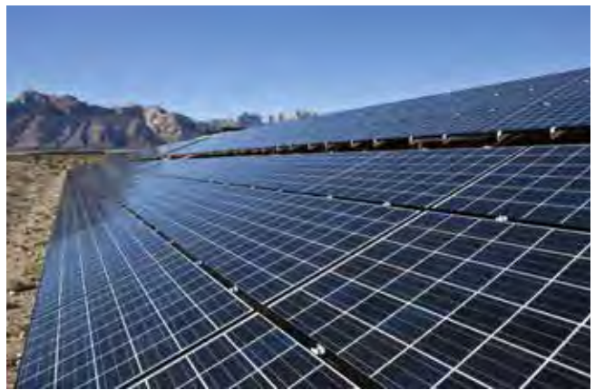
MEXICO Solem I & II, 175 + 165 MW HEC V1500 + MV SKID
